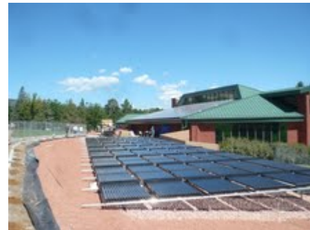
Boulder Rec. Center's solar-thermal project harnessing the power of the sun!
